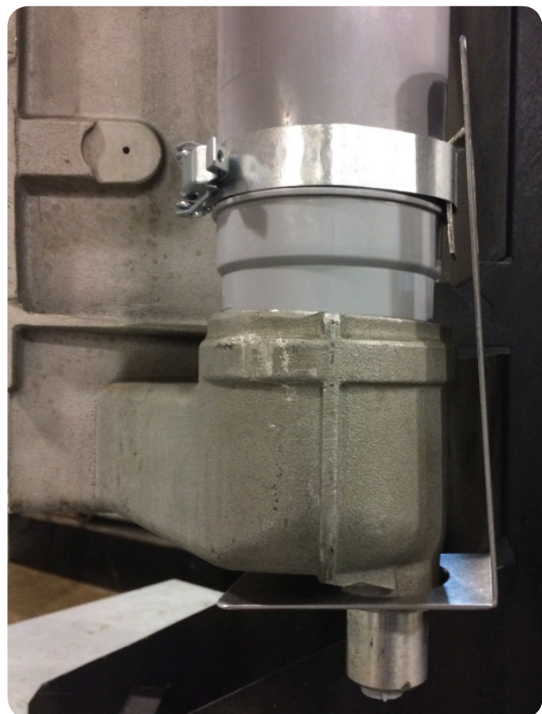
Figure 11 L bracket slid over condensate drain
